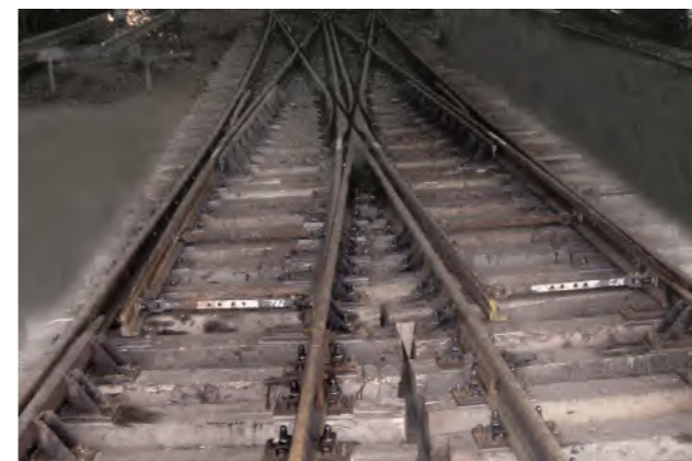
60kg/m Rail 1:7 Double Slip Turnout For Industry & Mining & Special Railway Line
